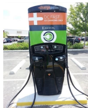
Figure 8. Dual-port DCFC station.
