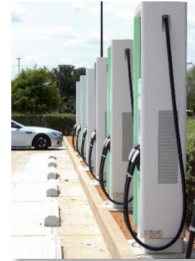
Figure 5. Electrify America station powered by CPS Energy.
