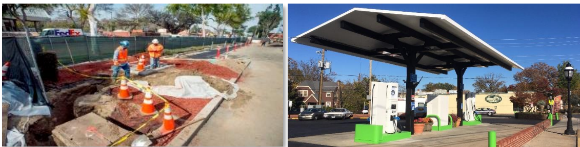
Figure 2. Installing and maintaining the estimated 10,000 charging ports needed by 2030 will create new jobs for electricians and construction workers.
